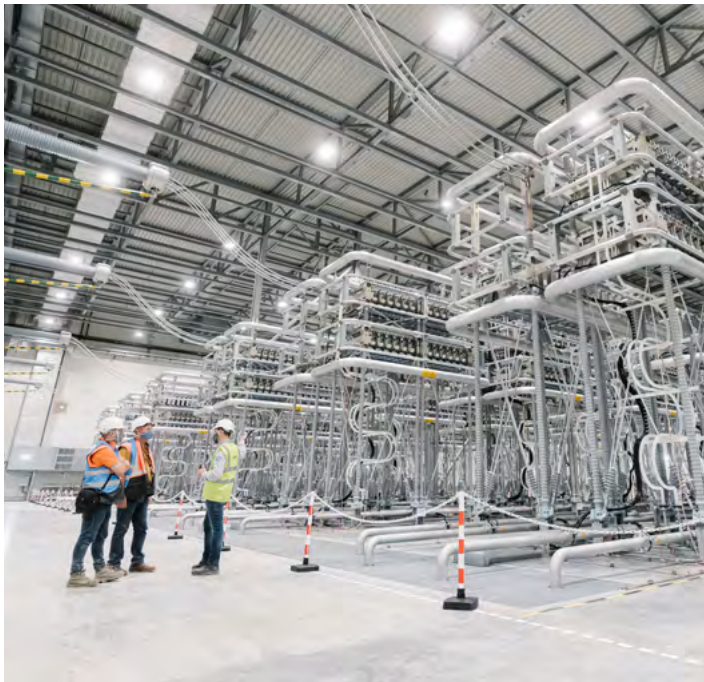
Interior of a converter station
