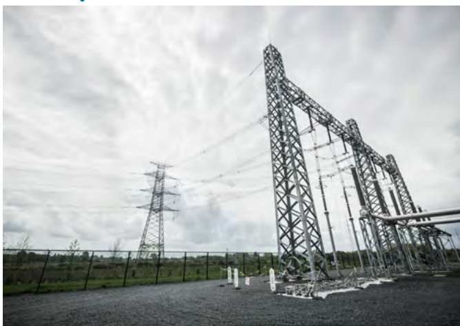
Connections in a high-voltage substation
