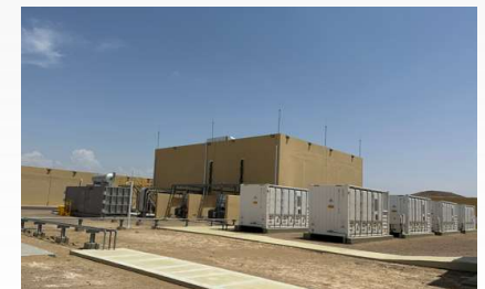
Site SD in stable operation
