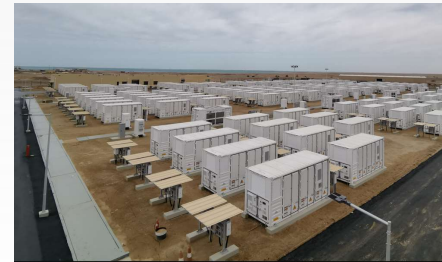
Site SF1 in stable operation
